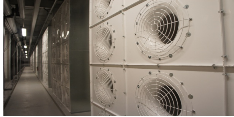
15 motors per server bank
